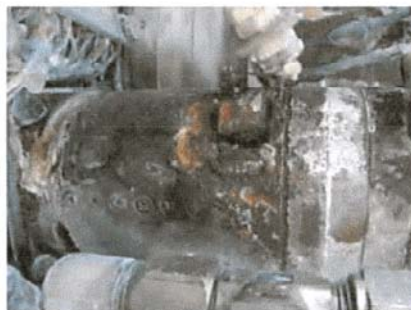
Picture 2: electrical connectors and cable as found after fire extinguished.
