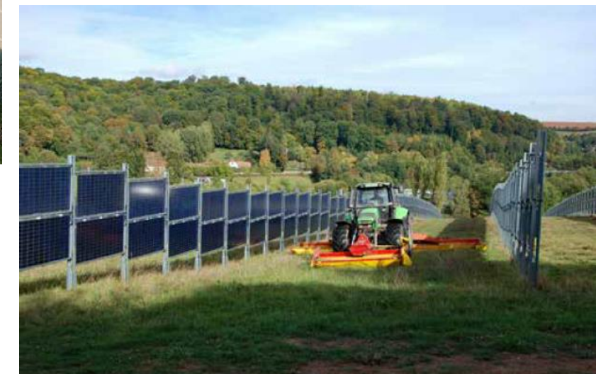
Impianti con moduli fotovoltaici bifacciali montati verticalmente su strutture fisse in the Eppelborn-Dirmingen solar park, Saarland, with 2 MWp capacity, constructed by Next2Sun GmbH. © Next2Sun GmbH
